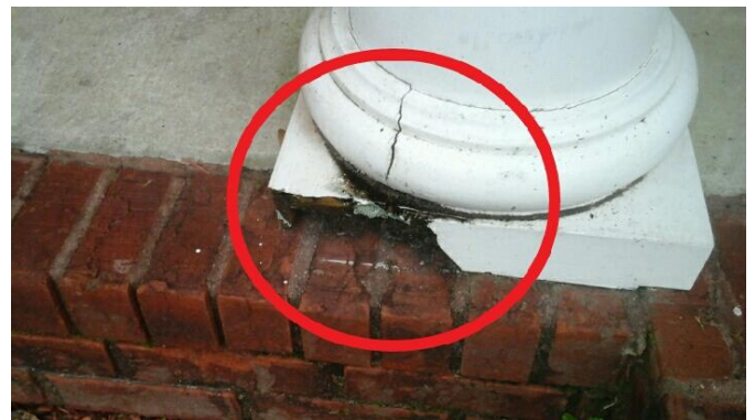
Repair as needed
